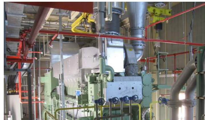
Inside view of Enclosure(Pre-fabricated type)
