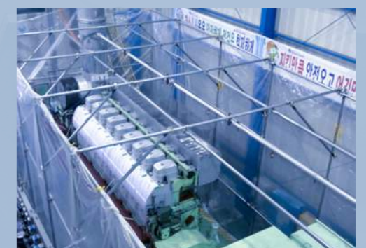
Water Spray Test for Kori #1 EDG
